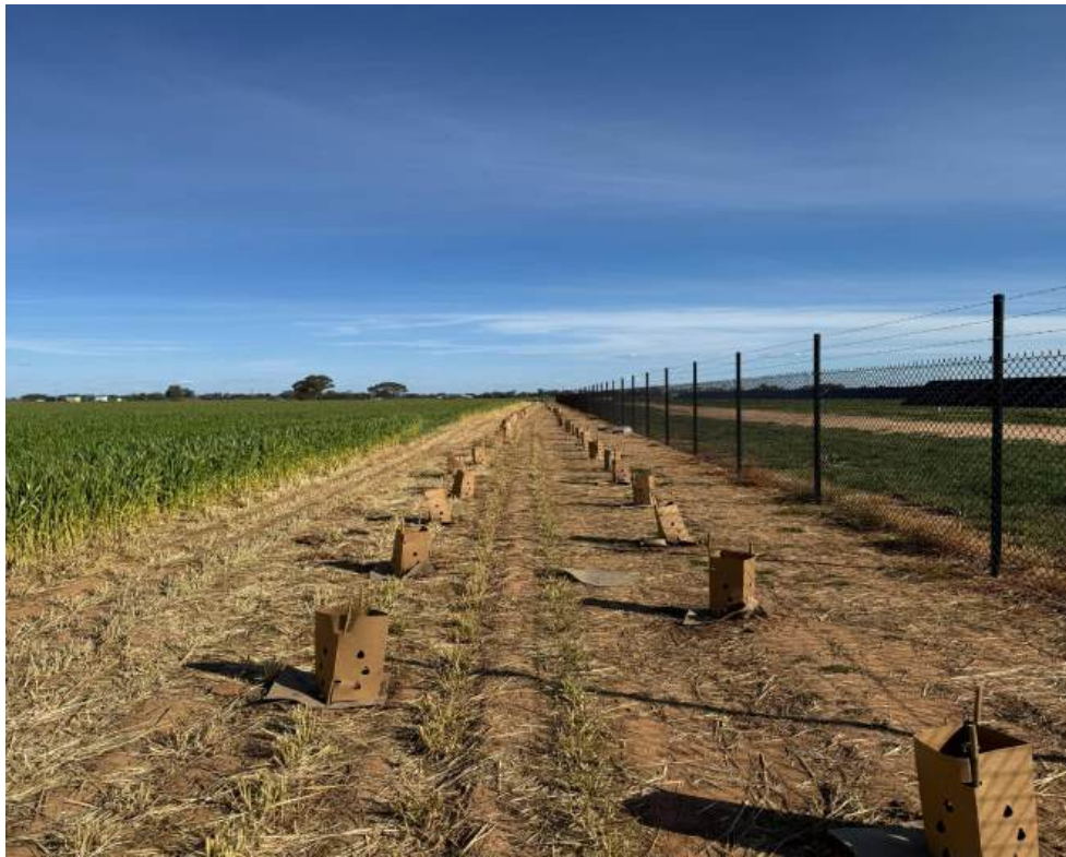
A new treeline for screening a solar farm in Narromine. The client stipulated the use of bioguards as protection. Photo: Jesse Powell
